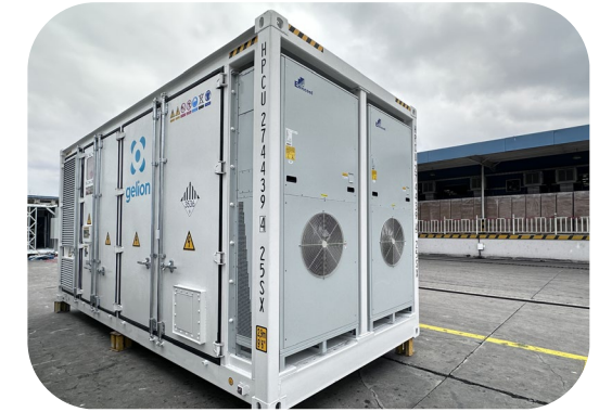
Containerised BESS currently in transit
